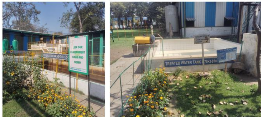
Figure 22. Effluent Treatment Plant
