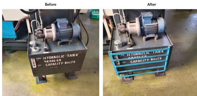
Figure 25. Reduced Hydraulic Oil Leakage
